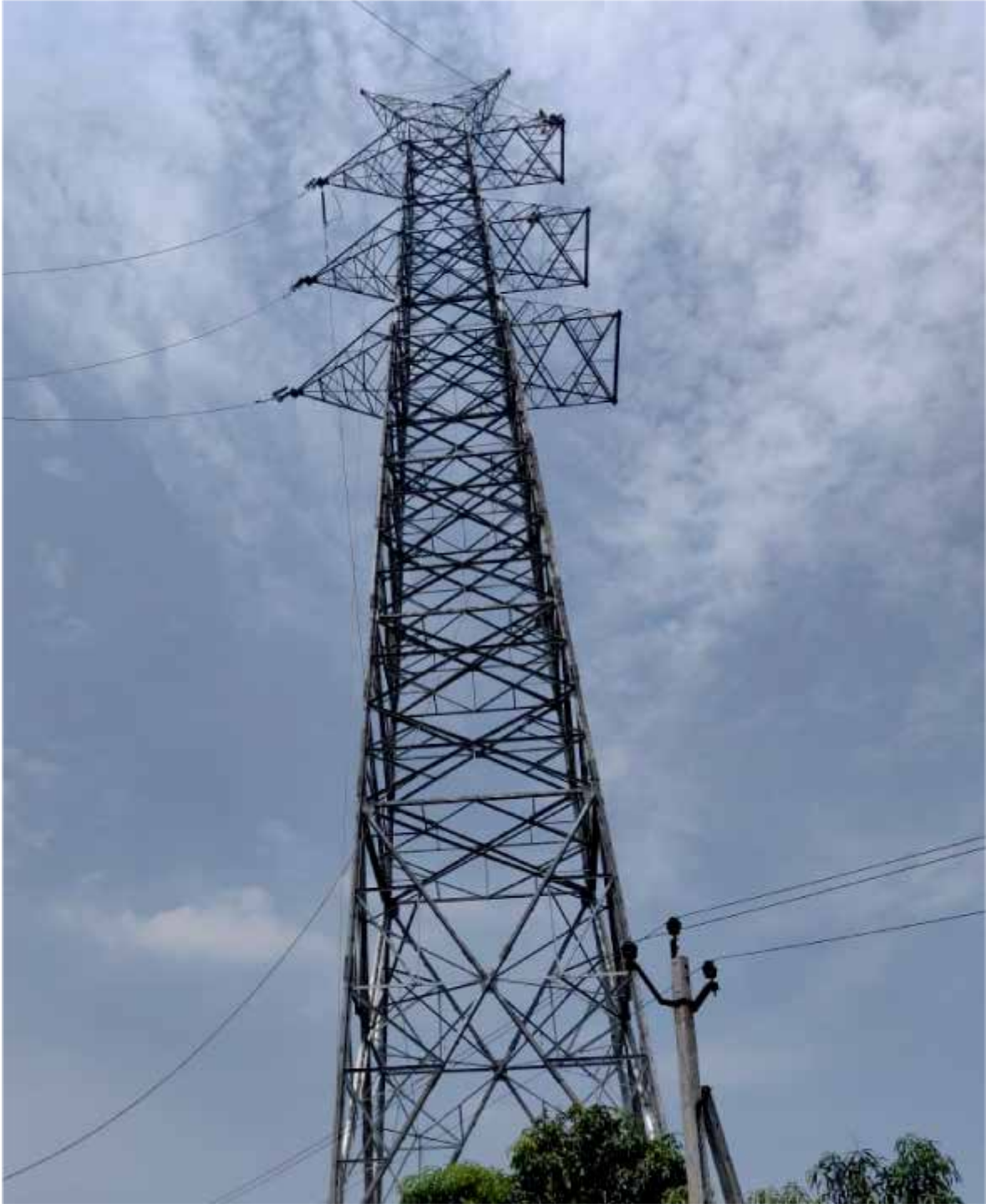
High-tension power cables and towers were shifted in order to make way for MAHSR corridor
