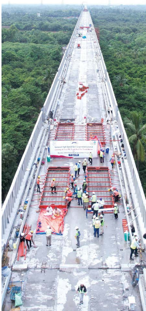
Tracklaying on the Mumbai – Ahmedabad high speed line started near Surat in August.
