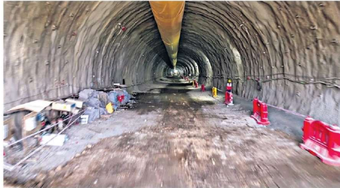
The 394-m-long intermediate tunnel, which has been excavated for the Mumbai-Ahmedabad Bullet Train Project, in Mumbai.
